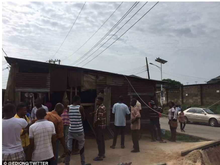
Fig 5. High- tension line fell on the roof in Calabar, Nigeria
