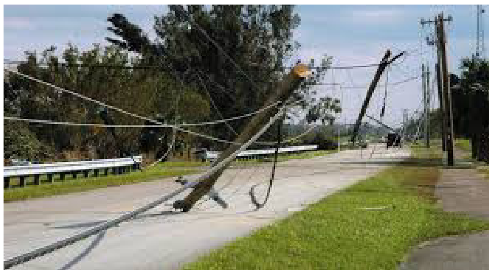
Fig.6.Damage high tension pole
