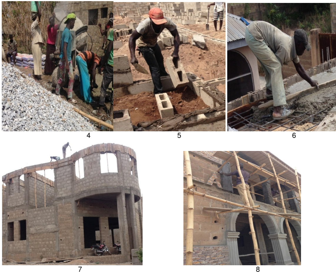
Figures 1 – 4: Awkward working postures of labourers at work Figures 5 – 8: Awkward working postures of bricklayers at work
